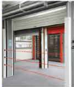
Motorised Shutters Safety Beam Sensor
