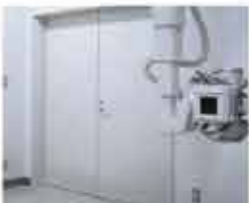
Insulated Fire Steel Door
